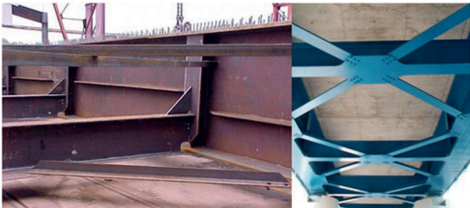
Figure 16. View of the bracings during construction (left) and for the finished bridge (right).
