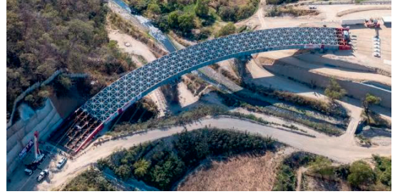
Figure 2 Overall view of the steel girders and bracings just after completing their construction. Source: PEDELTA
