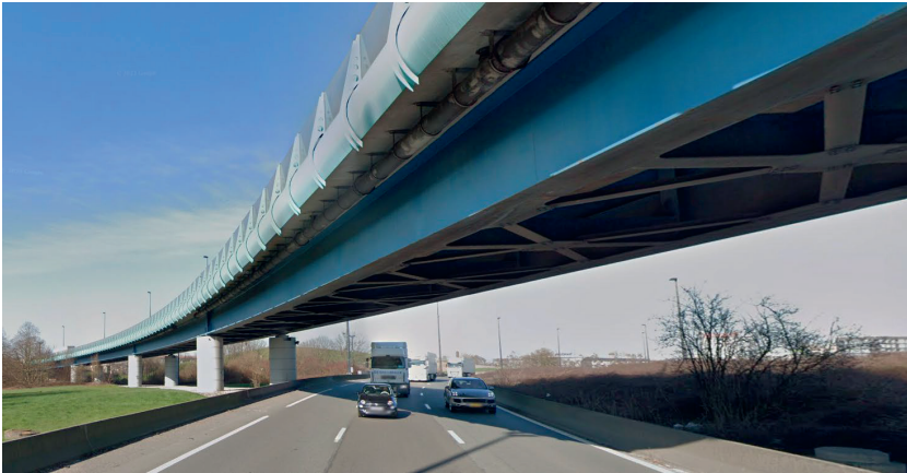
Figure 24 Street view from below on the Lille Porte Sud Bridge, (Google, n.d.).
