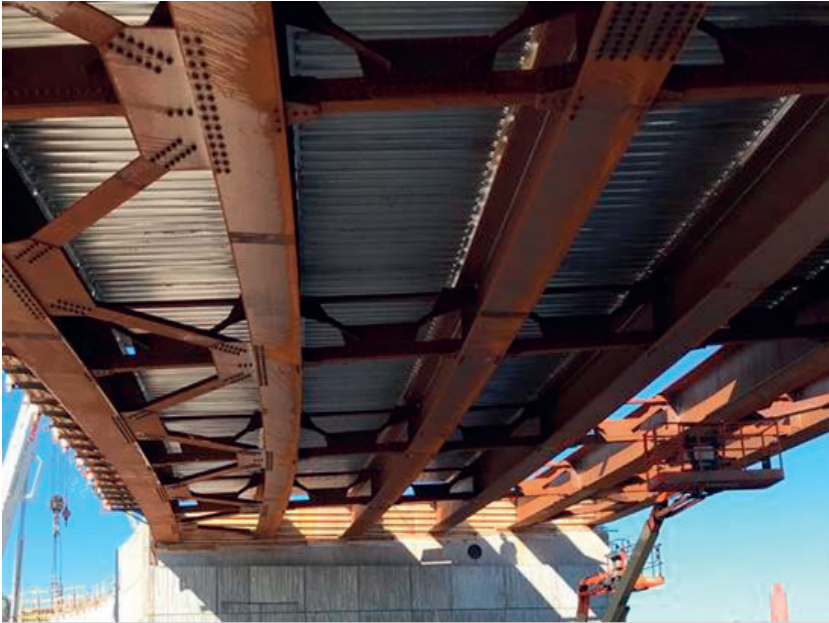
Figure 26. Bridge from underneath visualizing the multiple girders, cross bracing and lateral bracing at the outer bays. Source: Harry White
