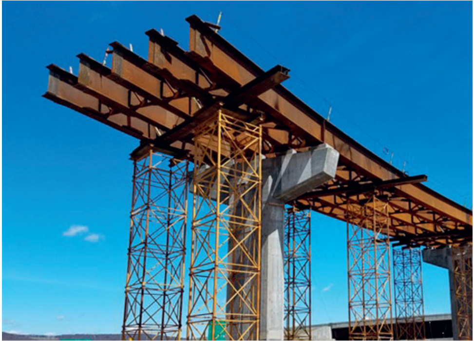
Figure 11. Bridge during the construction stage. The multi-cell modular joint is just out of view to the right.
