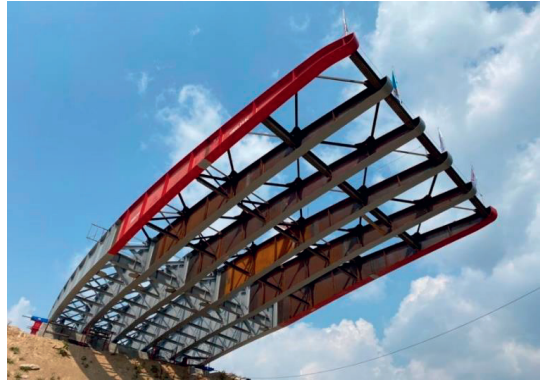
Figure 5 View of the bridge during launching, including the launching nose. Source: PEDELTA
