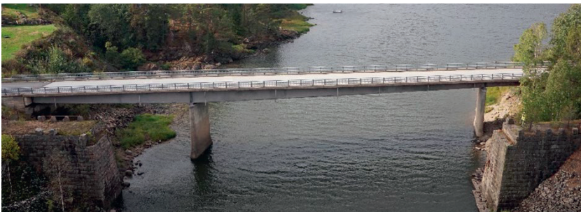
Figure 30. The Østre Trøsken Bridge, overview of the bridge from north (Paper II / Vestman et al., 2022).
