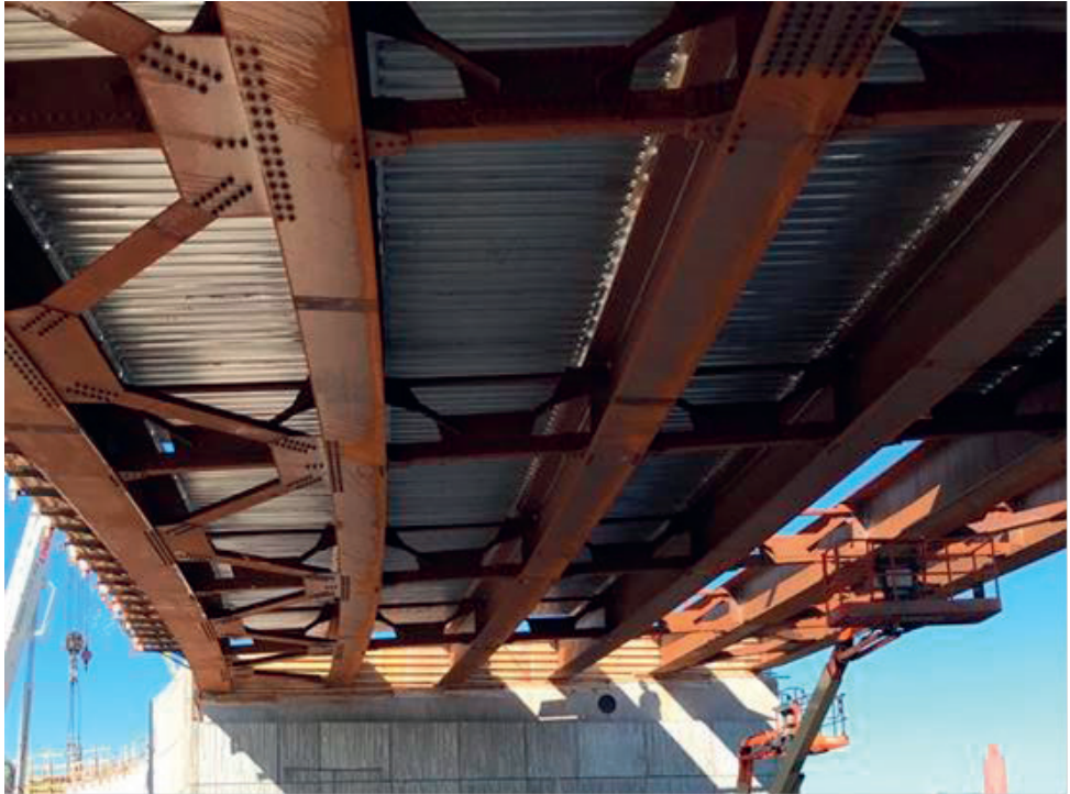
Figure 10. Horizontal bracing located only in the exterior bays and stay-in-place forms visible between the girders.
